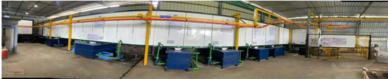
8 STAGE SPRAY PRETREATMENT LINE & WATER DRY OFF OVEN
